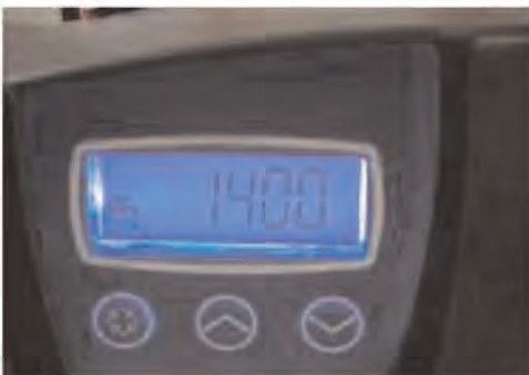
Fig 5 Remaining gallons to backwash. Ecosmarte® Control Valve is displaying the remaining gallons to backwash, as indicated by the red LED display.
